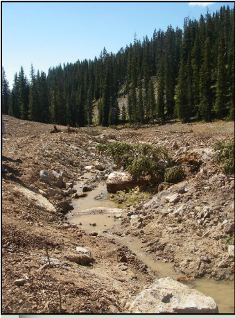
Above: The Forest Service and EPA redesigned the channel for Elk Creek. Sedges, willows, and other vegetation were planted as part of the revegetation of the site.
